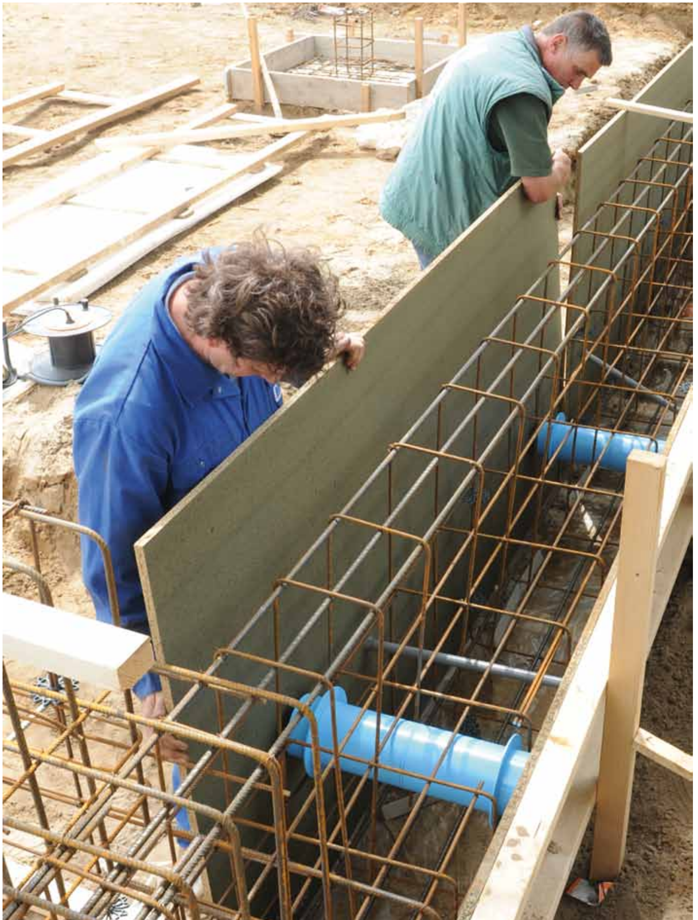
The casing plate at the other side is provisory placed to enable marking the position of the fixation pieces.
