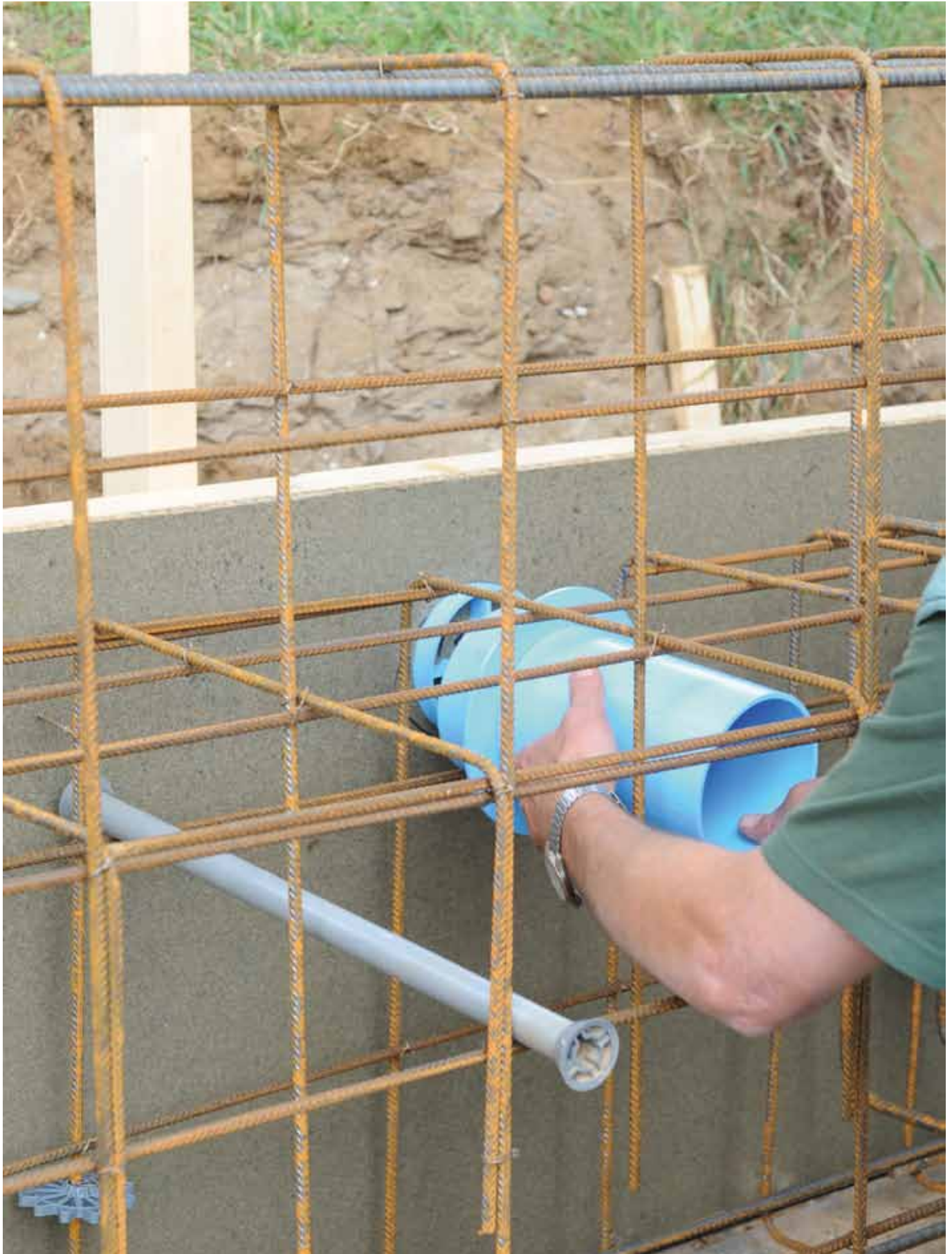
The conduit inlet with an adapter pipe is placed over the fixation piece.
