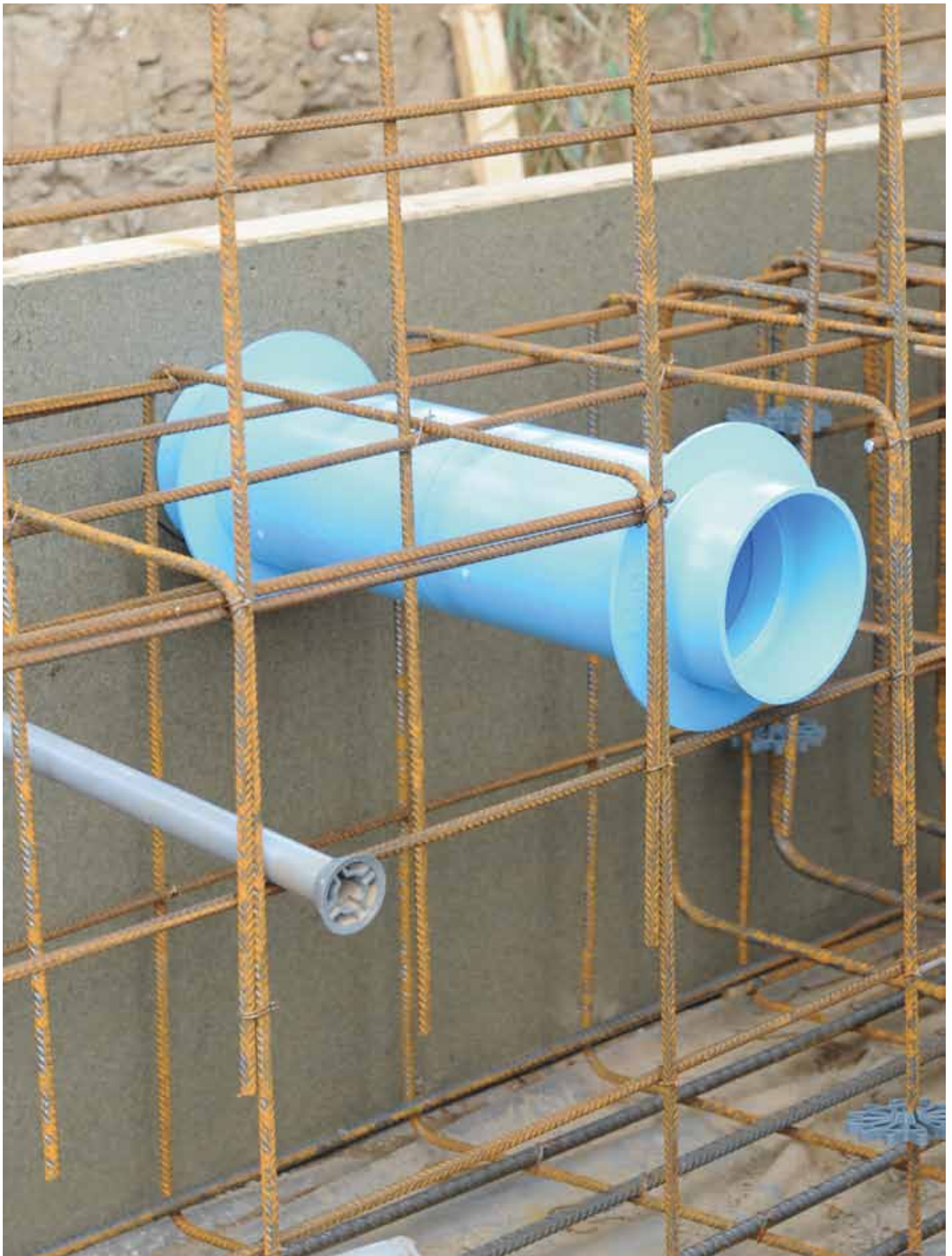
Positioned embedded pipe inlet in between the steel armouring of the foundation to be cast.
