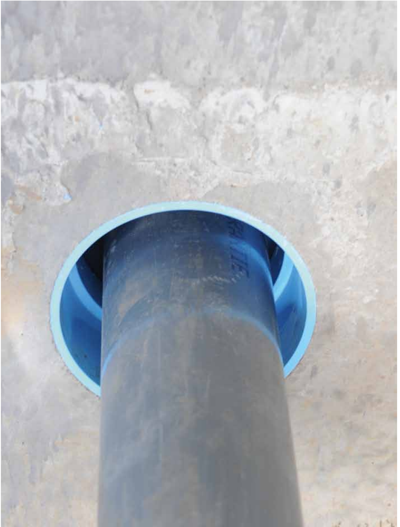
PVC pipe ducted. Conduit inlet is 125 series; the PVC pipe has an OD of 90 mm.
