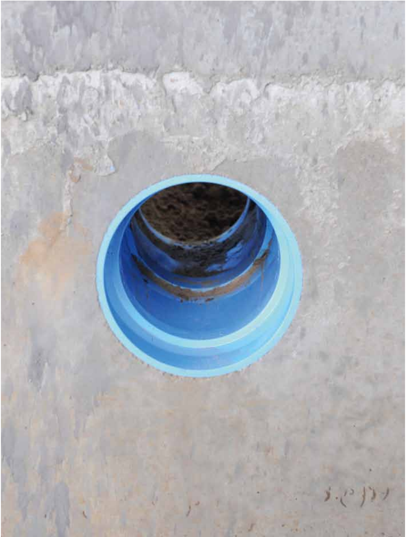
The conduit pipe inlet system after casting the concrete and removal of the casting plates. Due to bad weather some mud is visible inside but there are no concrete residues visible.
