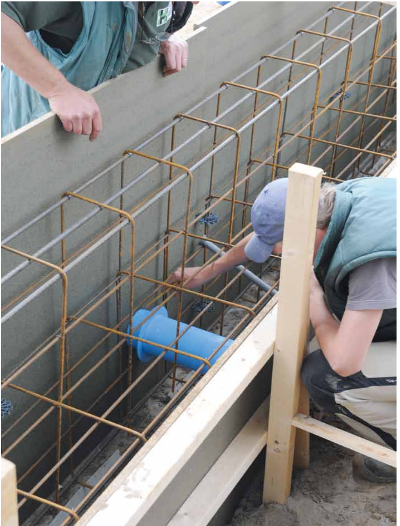
The contour of the conduit inlet is marked on the casing plate.
