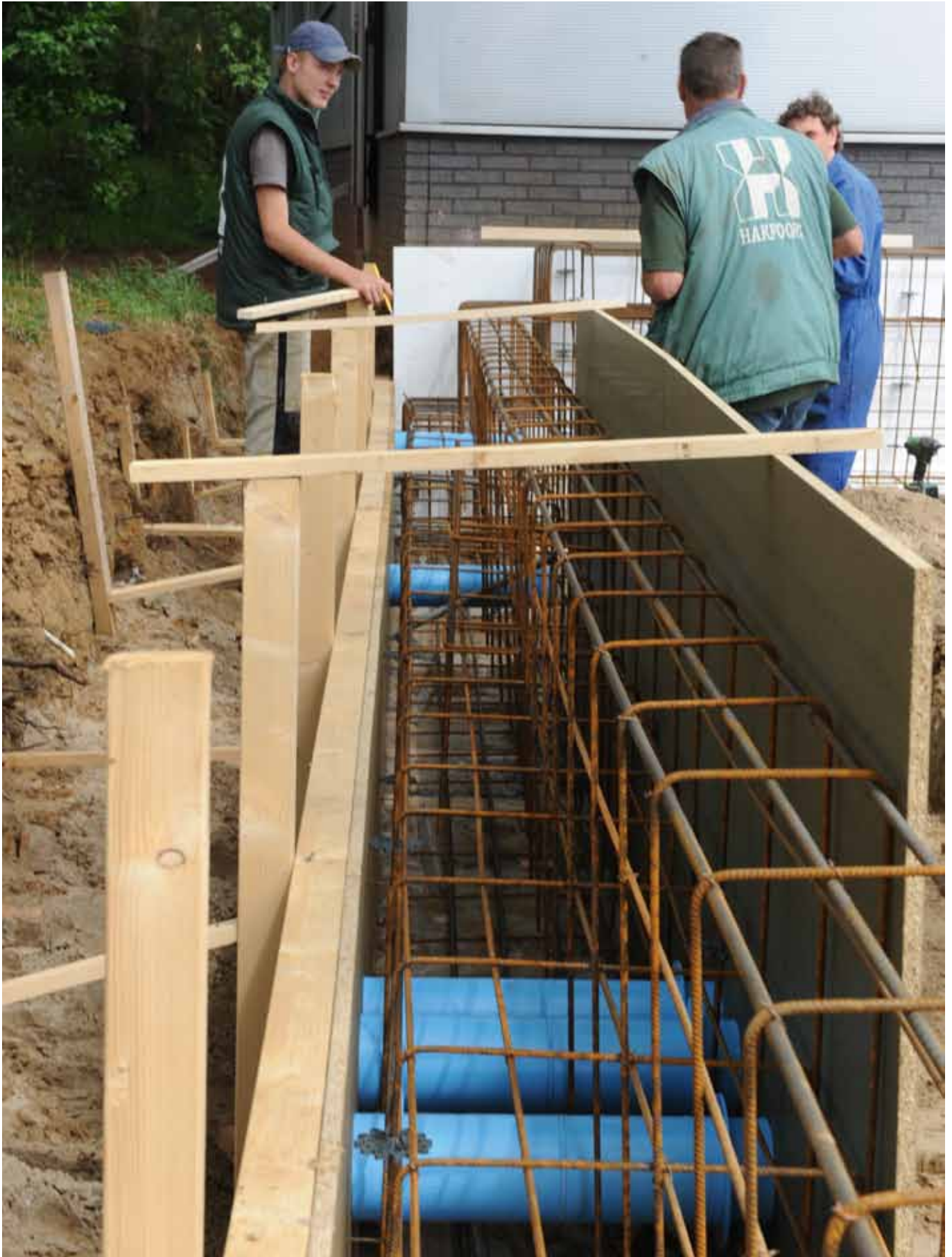
Overview of the embedded pipe inlets placed at this part of the construction.
