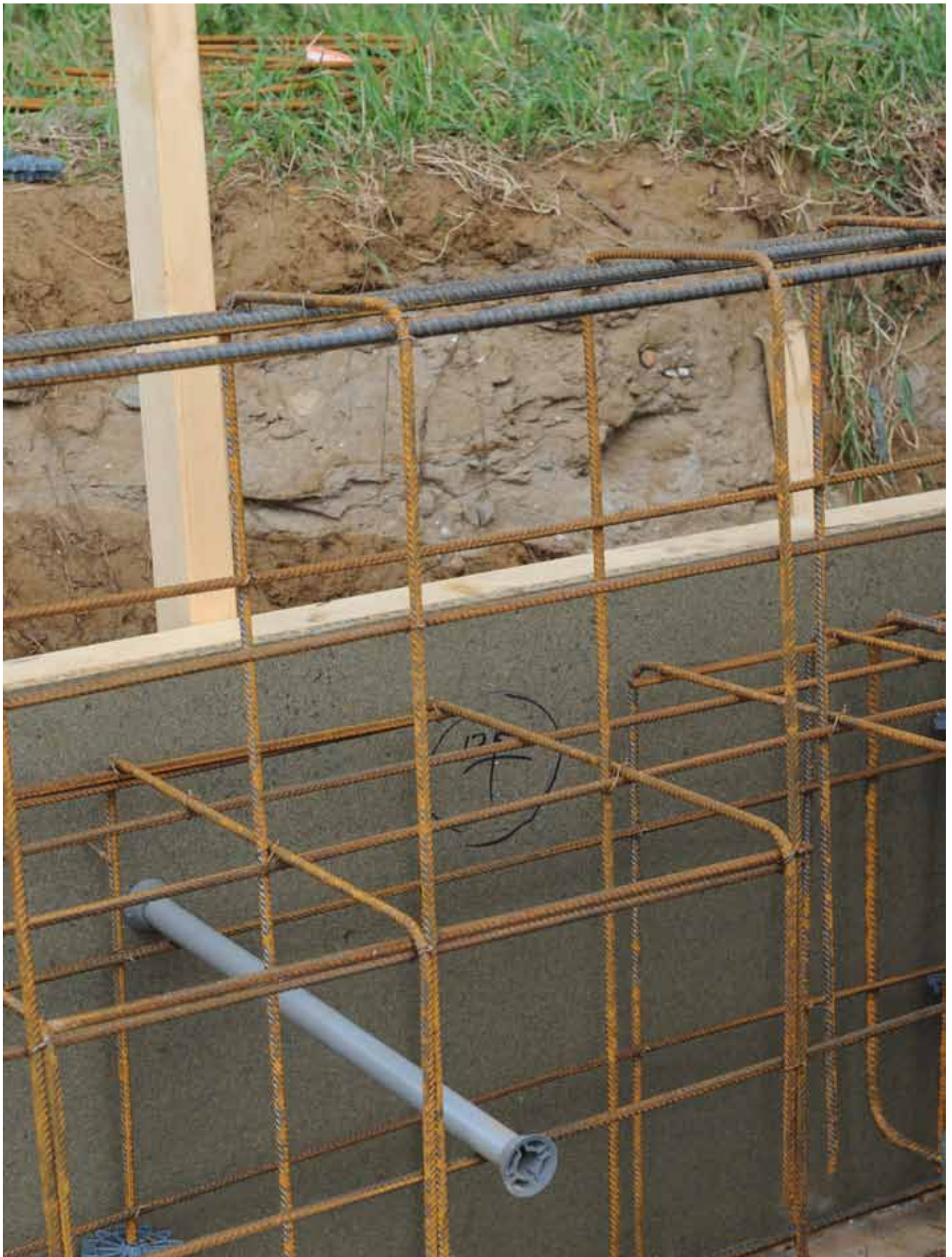
The position of the 125 mm inlet is marked on the plating of the casing prepared to cast the concrete.
