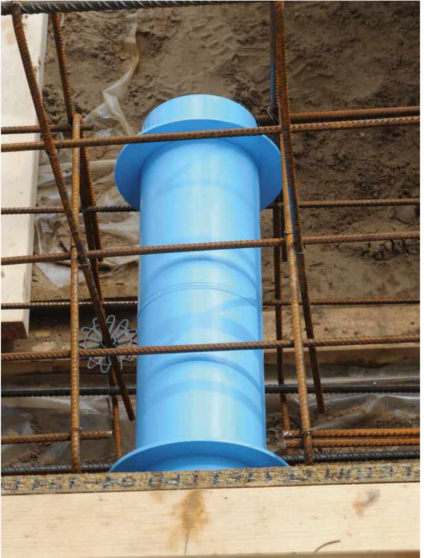
Close-up of the set. One of the adapter pipes has been cut to size.
